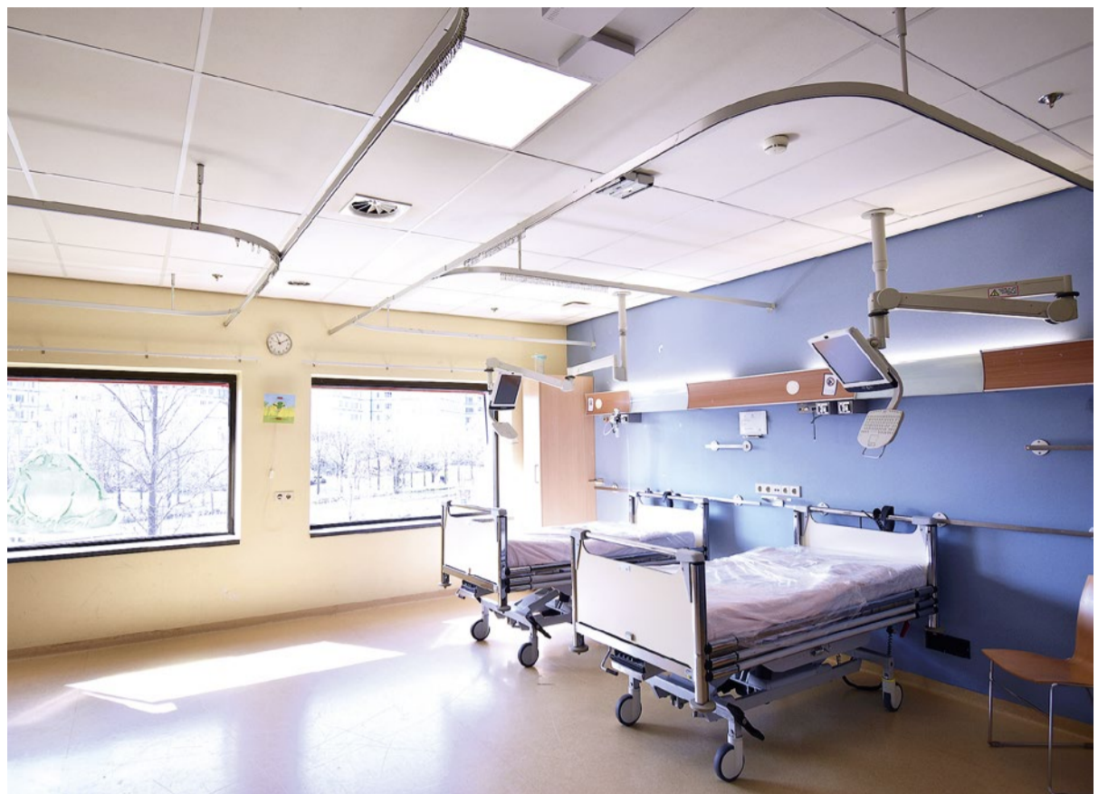
Hospital ward features track/trace tags on beds and intelligent lighting
